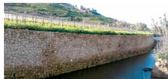
Construction of the rubble walls at Ramla Valley in Gozo in the framework of the Alter Aqua Programme, September 2013.
